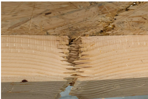
FIG. 5. Close-up of the damage area of the beam from Fig. 4.
