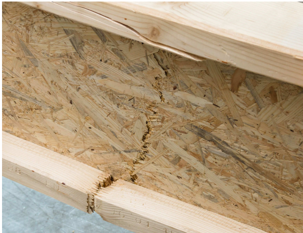
FIG. 4. Destroyed connection in tensile wooden flange.
