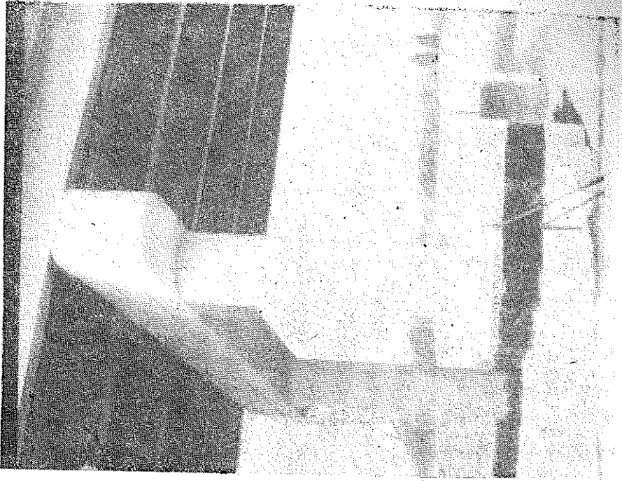
FIG. 9. Steel barrel system protecting bridge abutment.
